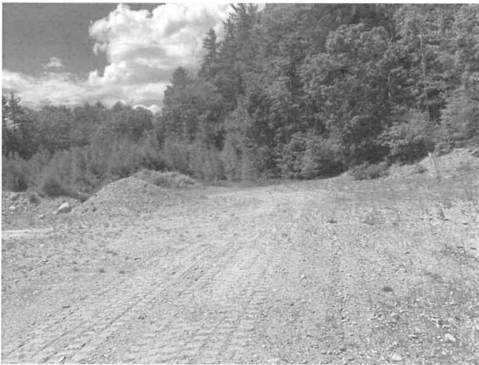
Photograph No. 6: Looking across the Site from the northeastern portion of the Site.
