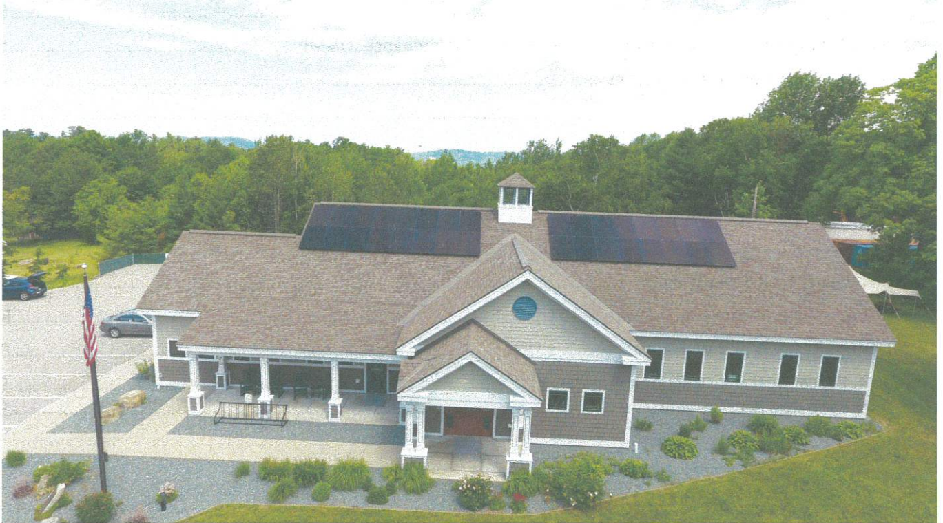
Recent Mains Electric installation at the Bethlehem Public Library
