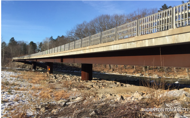
New Hampshire DOT, Bridge No. 239/152, NH Route 49 over the Mad River, Thornton, NH
