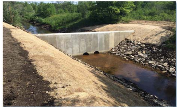
Outfall Slope Stability, Rockland, MA
